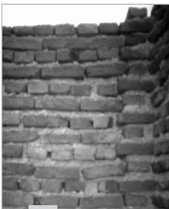
Figure 3.12: Improper bonding of masonry units
