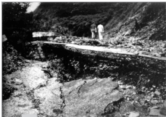
Figure 3.4: The damage of road in Koshi Highway
