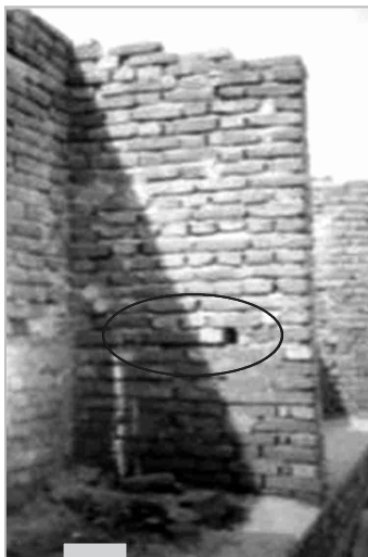
Figure 3.9: Weakness in building construction
