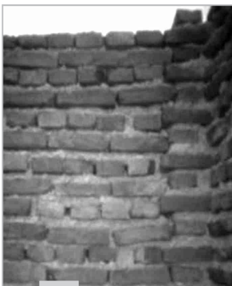
Figure 3.12: Improper bonding of masonry units
