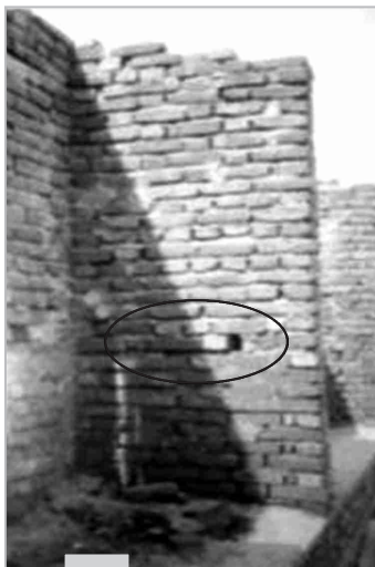
Figure 3.9: Weakness in building construction
