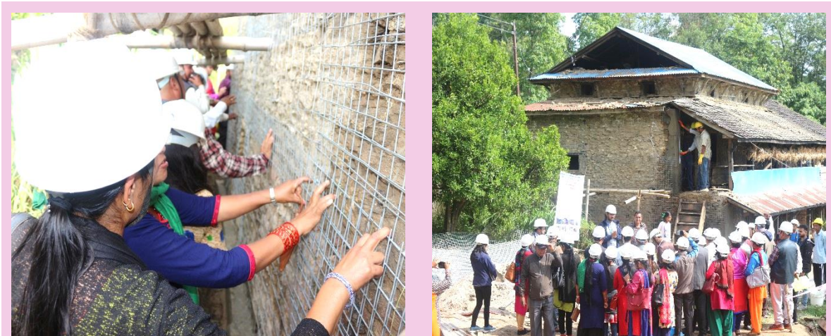
Figure 4. Local community people including house owners, local government representatives and others visiting a demonstration construction site on retrofitting to learn about the technique. Such demonstration visits were facilitated by Baliyo Ghar Program through awareness campaigns or trainings.
