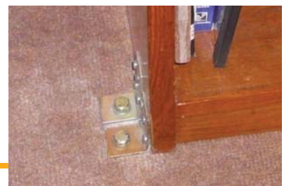
Non-structural Mitigation: Anchor bolts fixing book rack to RC floor below Source: NSET
